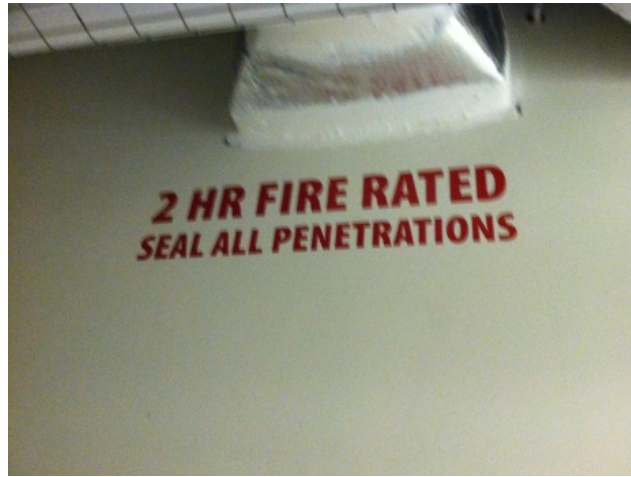
Photo 1 – Fire Wall Label Example #1
