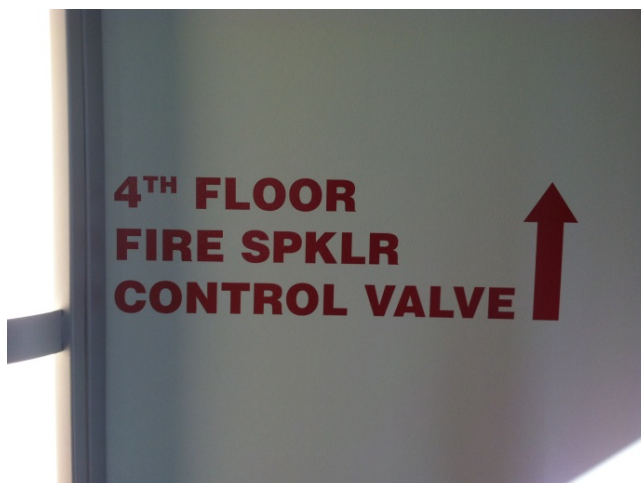
Photo 3 – Floor Control Valve Identification
